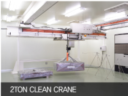
2TON CLEAN CRANE
